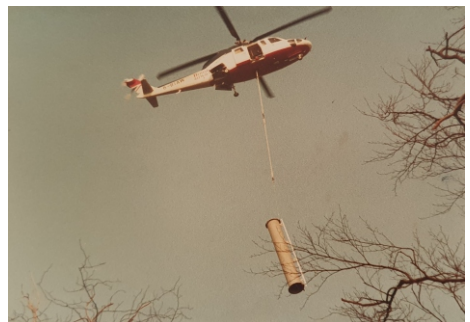
A photograph of the daring engineers installing the tower pylon by helicopter in 1984.
